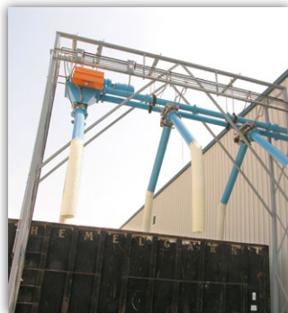
Discharge end of the 400 ft (122 m) tubular drag conveyor. Each discharge has a bi-directional gate.
